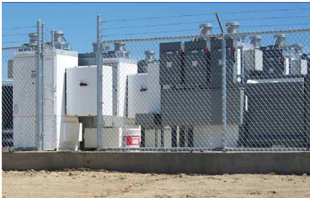
Figure 74. Utility-scale inverters use higher DC input and AC output voltages to reduce losses, and the size and costs of the conductors and switchgear required.
