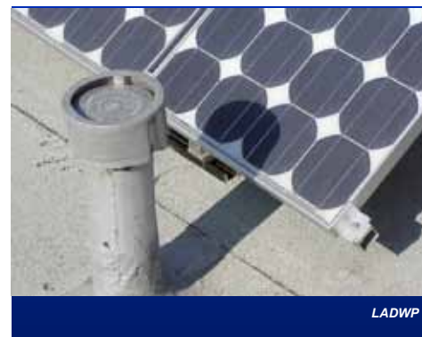
Figure 17. Shading of PV arrays can be caused by any obstructions interfering with the solar window.
