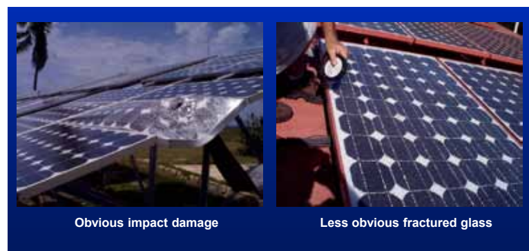
Figure 109. Inspect PV arrays for any signs of physical damage, such as impacts or fractures.
