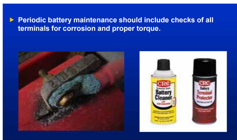
Figure 115. Periodic battery maintenance should include checks of all terminals for corrosion and proper torque.
